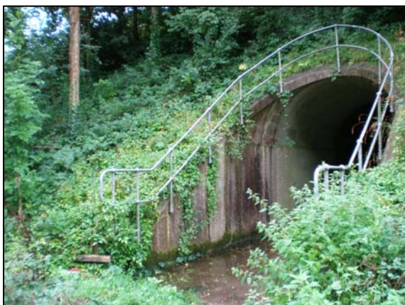
Undergrowth surrounding the tunnels causes water to run onto the concrete floor.
