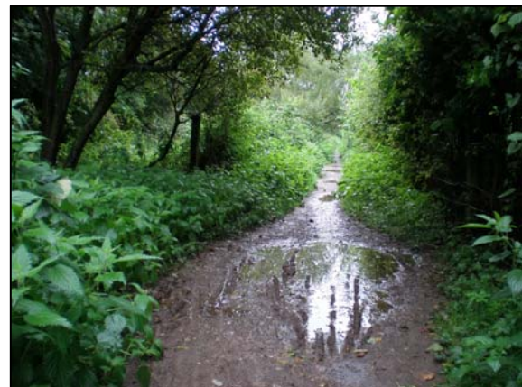
Deep potholes need filling, and a new layer of hard surfacing needs to be spread along the path.
