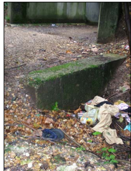
Litter in the storm drain between the A34 tunnels.
